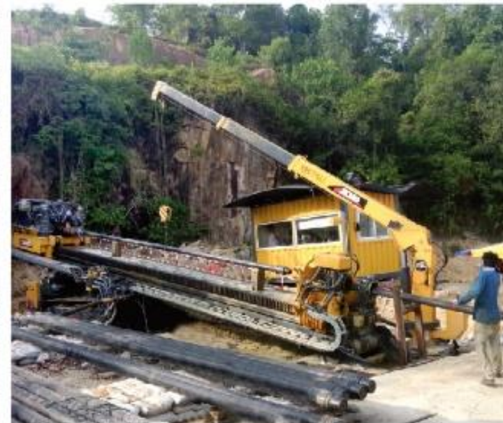
XZ5000在马来西亚穿越卢穆特海湾 XZ5000 works to get through Lumut Bay in Malaysia
