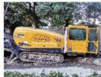
XZ420E水平定向钻机泰州电力管道项目施工 XZ420E HDD is working for the electricity pipeline project in Taizhou City
