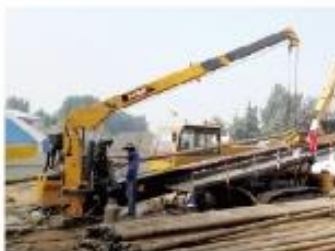
XZ3600水平定向钻机在山东泰安施工 XZ3600 HDD working in Ta'an Shandong
