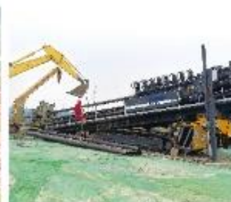
XZ13600河北唐山曹妃甸双龙河穿越工程施工 XZ13600 HDD is working to get through Caofeidian Shuanglong River in Tangshan City
