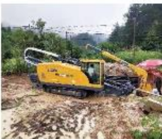
XZ960E江西管道项目施工 XZ960E HDD is working for the pipeline project in Jiangxi Province
