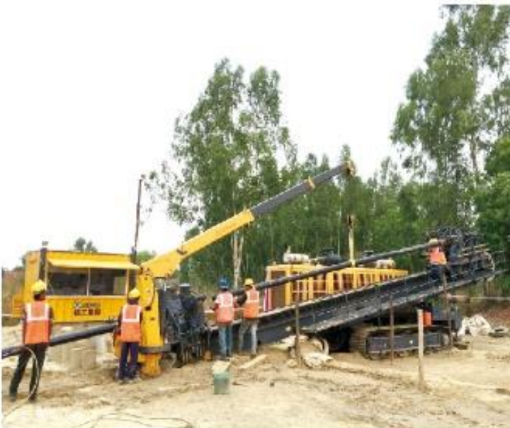
XZ3000在印度坎布尔穿越恒河2.2公里 XZ3000 HDD works to get through Ganga River by 2.2Km Kanpur
