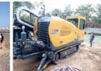
XZ360E水平定向钻机在河南郑州施工 XZ360E HDD works in Zhengzhou City, Henan Province
