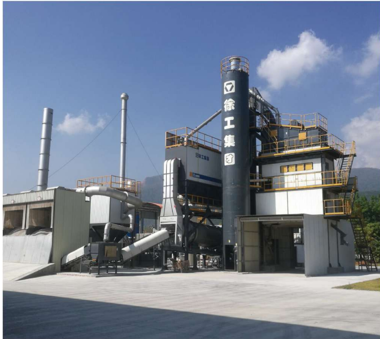
徐工环保型沥青站云南瑞丽施工 XCMG environmentally-friendly asphalt plant in Ruili, Yunnan province
