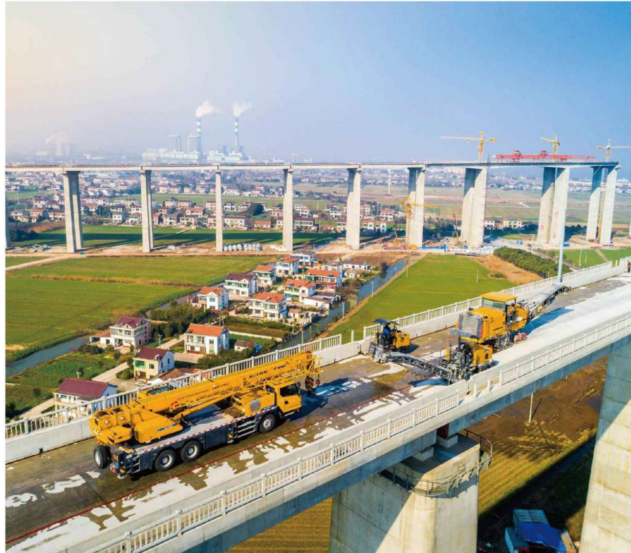
徐工铣刨机组助力世界最大跨度公铁两用斜拉桥 XCMG milling machine helps the world's largest span of rail and road dual-use flyover
