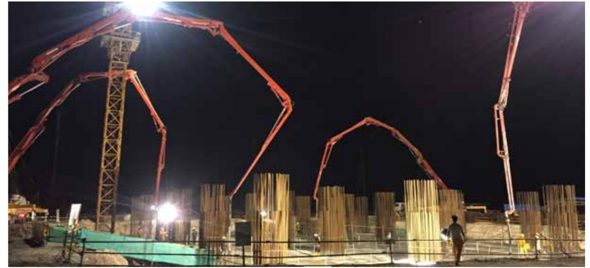
四蛟龙齐助尼日利亚建设 Four boom pump are cooperating like dragons in Nigeria
