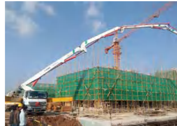
徐工HB52V泵车云南施工 XCMG HB52V boom pump is working in Yunnan
